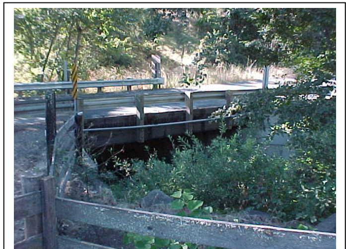
Figure 6. Upstream of Bridge 65C74 (timber superstructure, concrete abutments, vegetative growth in stream)
